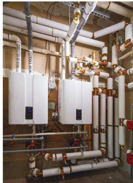
Two NHB-150 boilers were installed in each of 10 eight-unit apartment buildings.
